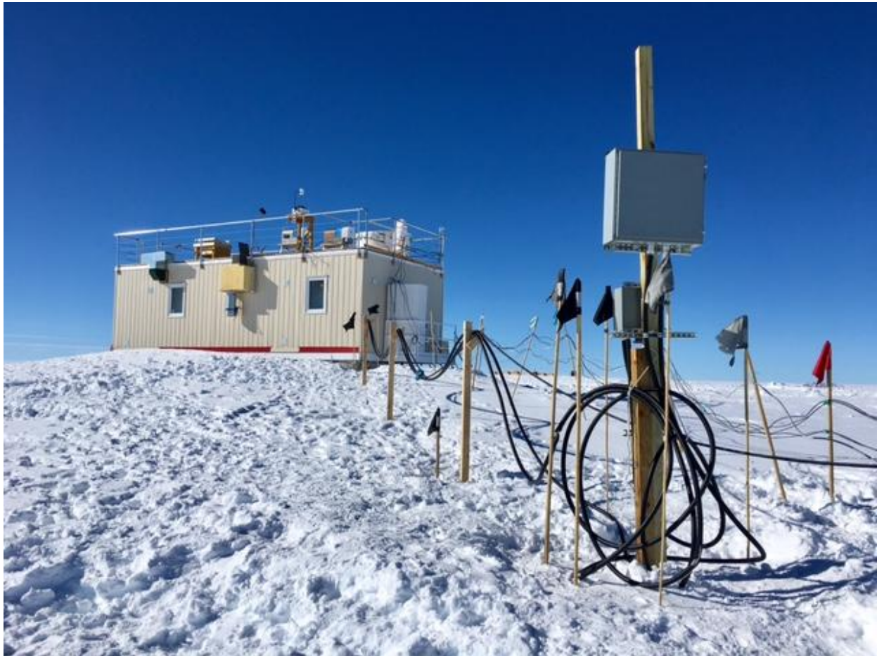
The MSF power boxes and cables were raised above the drift forming on the south side of the MSF. (Photo taken 07-11 by Marci Beitch)
